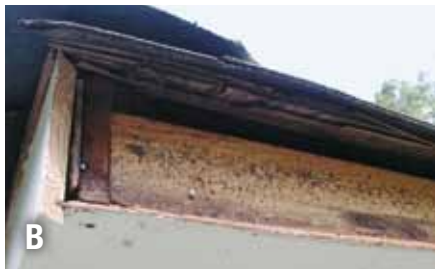
Figure 5. The structure itself is comprised of an almost endless series of voids and other potential harborage sites, such as (A) crawlspaces, and (B) the attic area behind fascia boards, where smokybrown cockroaches were living (the dark stippling is cockroach frass).
