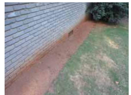
Figure 7. The area next to foundation walls should be kept free of vegetation.
