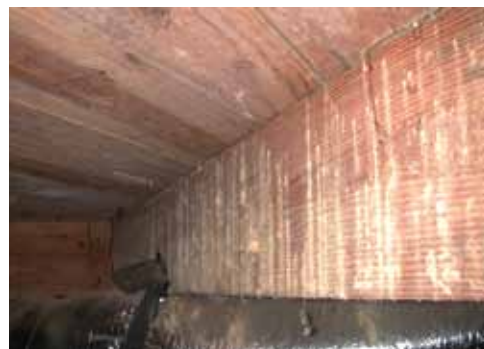
Visual evidence (frass streaming from exit holes) of an active anobiid powderpost beetle infestation in a crawlspace joist.
