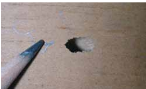
Wood-boring beetle exit hole
